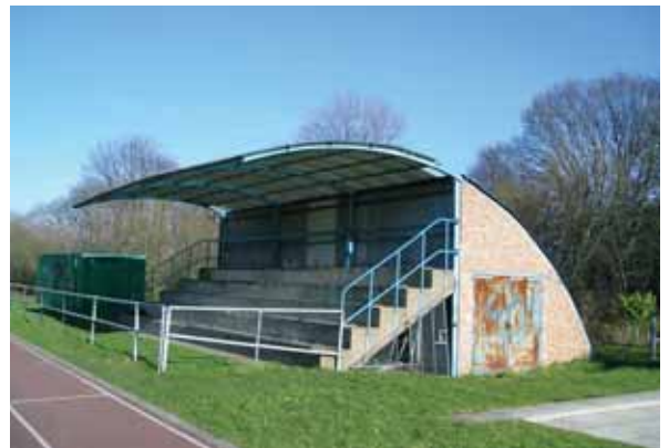
Stand in poor state of repair
